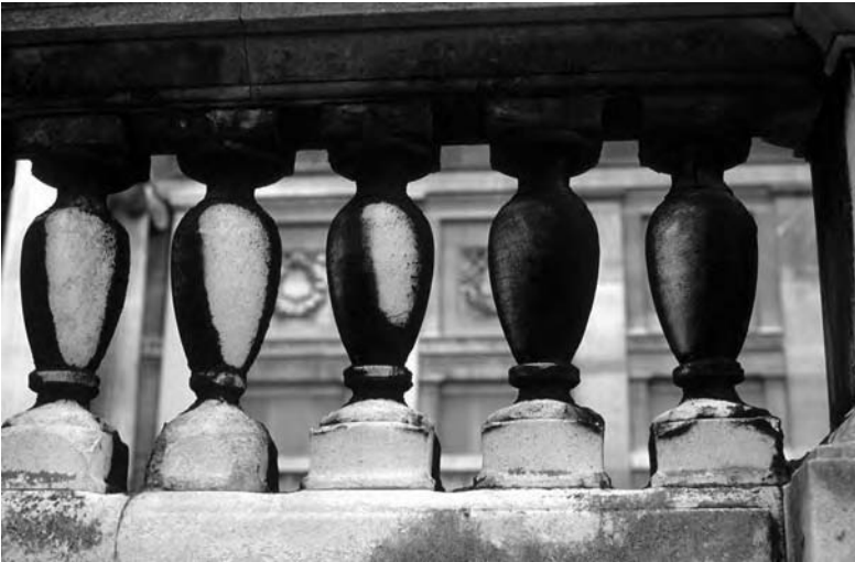
Plate 5.1 Weathered balustrade on the Ashmolean Museum, Oxford, England. The balustrade has now been cleaned.
